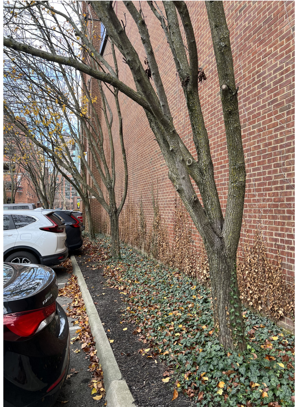
+/-6' plant bed on north side of North Bank Condos at Neil & Spring
