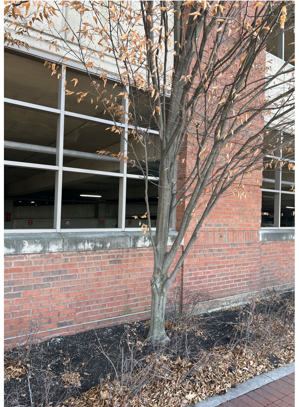
Same bed showing tree +/-2' off of face of building
